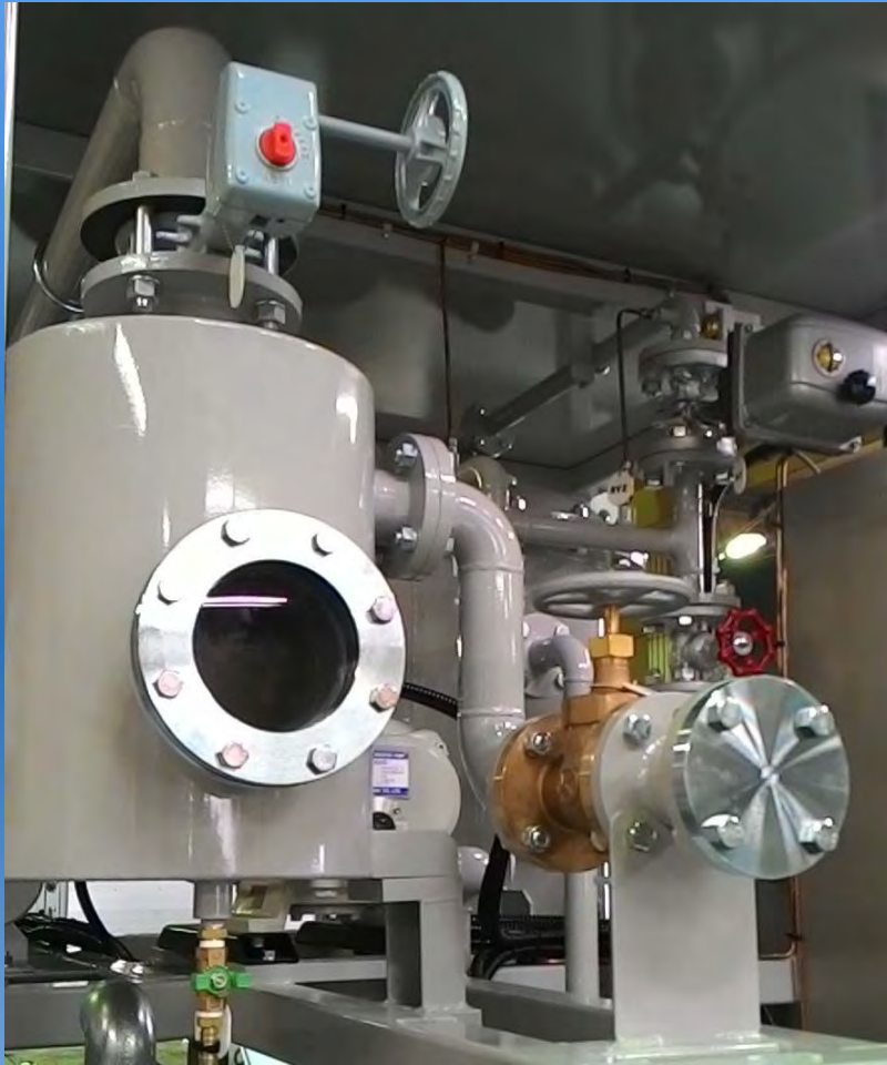
VACUUM PORT: Evacuate transformer
